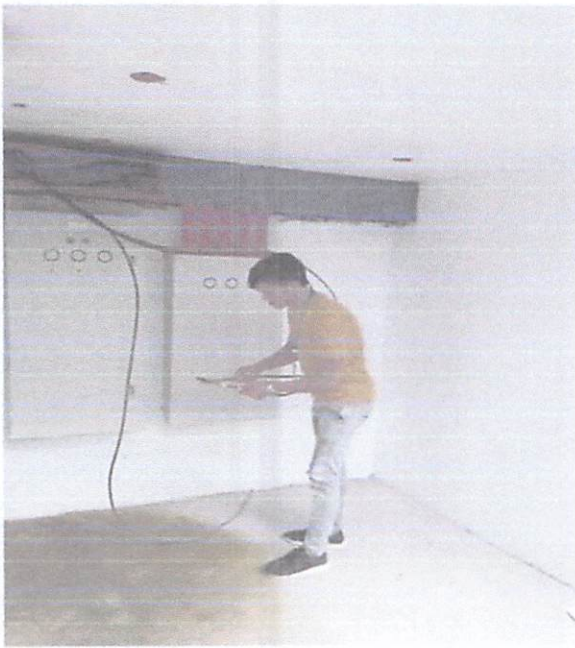
Fig. 02- Checking control panel
