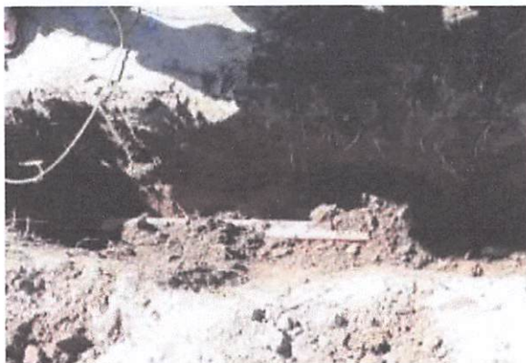
Figure 12: Buried plastic pipe
