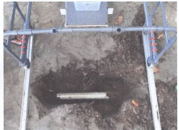
Figure 11: Buried metal pipe
