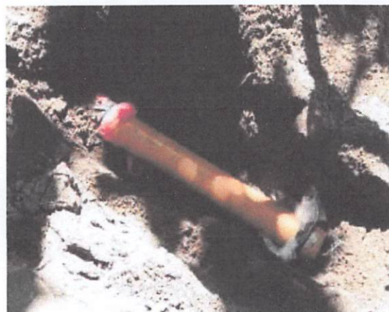
Figure 13: Buried plastic pipe with water
