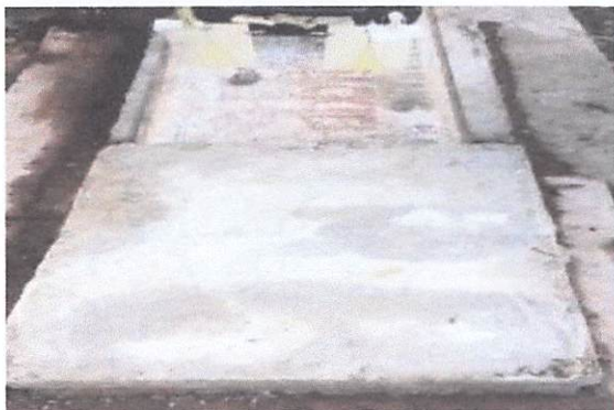
Figure 12. Concrete Slab with Void Space
